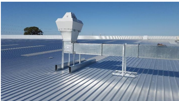
Commercial air conditioning
