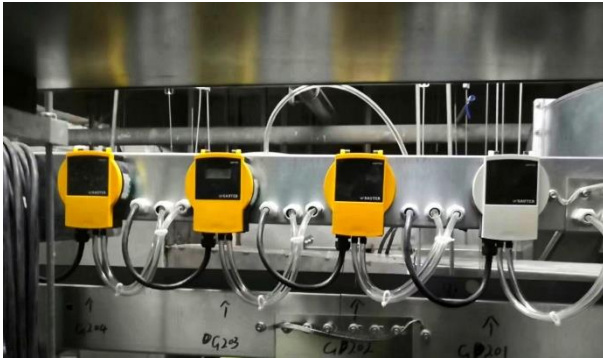
Image: SAUTER differential pressure transducers (EGP 100) for room pressure control and monitoring installed at the Sinopharm vaccine production plant
