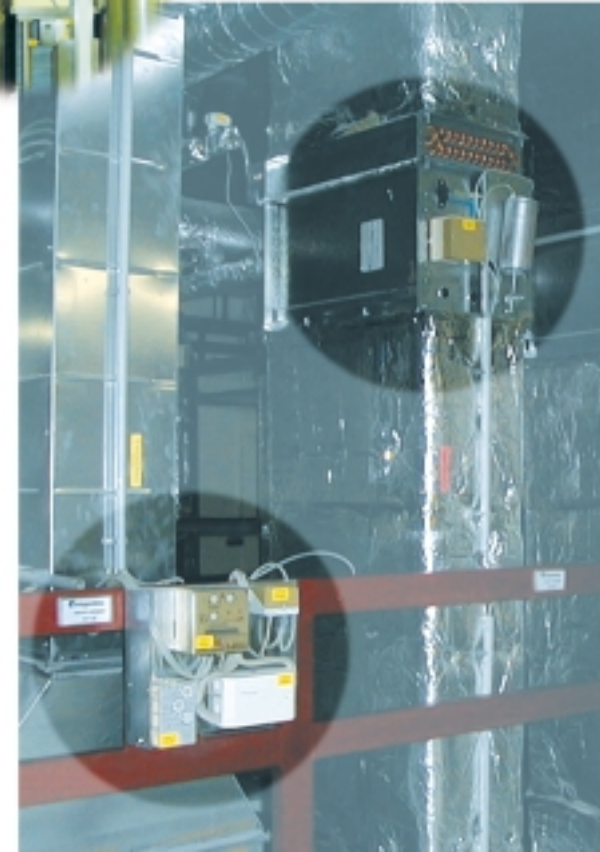
Air supply and extraction unit of a clean room area. Pneumatic-electronic controllers and converters are brought together in a single panel and linked through electrical as well as pneumatic circuits to the other measurement and control units.
